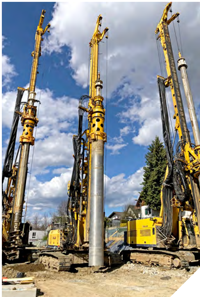
CONSTRUCTION OF THE APPROX. 700 PILES in just ten weeks with three machines
